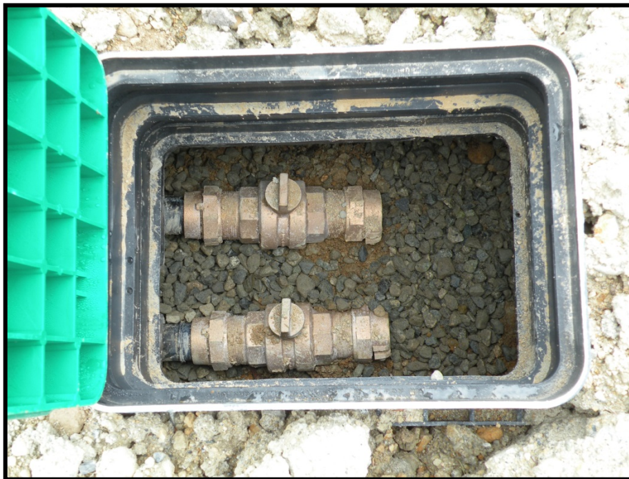
Figure 1: Curb-side valve box located near the property line of each home.
