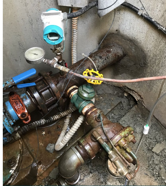
Well 3 Pump and Electrical Upgrades ($251K)
